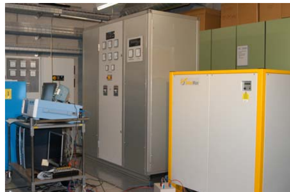
Figure 6: 100 kW solar generator simulator with a 100 kW inverter from Sputnik (photo: BFH-TI).
