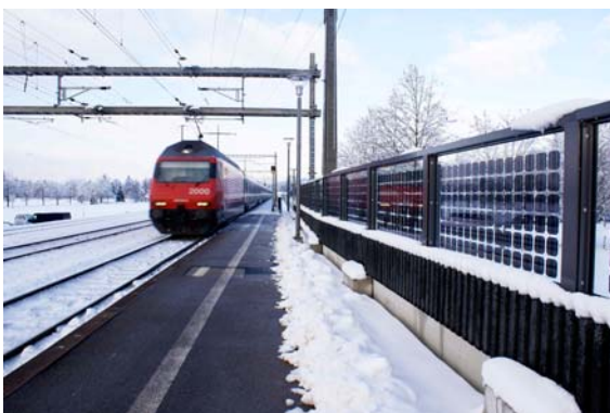
Figure 7: Bi-facial photovoltaic noise protection barrier (photo: TNC)
